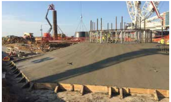
Cast-in-place foundation placed prior to casting pedestal wall and backfilling with soil
