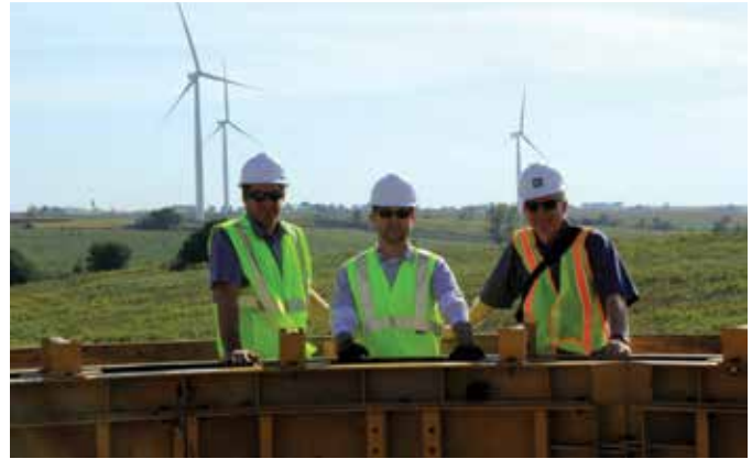
From left: Matt Chase, Steven McRory, and Jim Lockwood inspecting formwork prior to the next concrete placement
